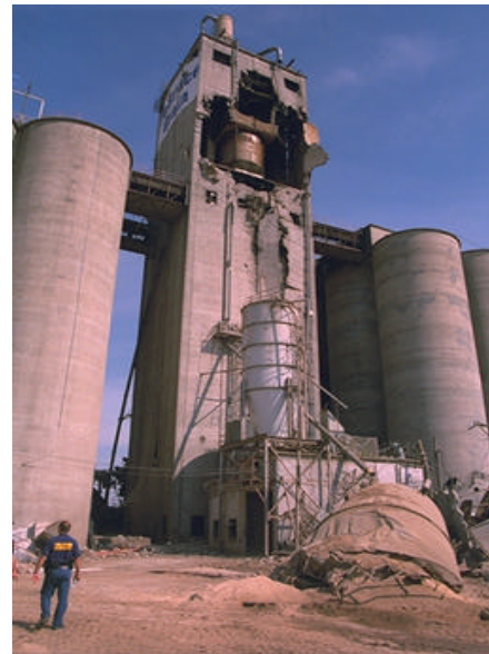
Figure 1: Photo showing damage to headhouse structure (NFPA)
